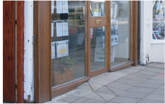
Picture 3 POOR : Stall riser
