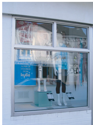
Picture 11 POOR : Mullions
