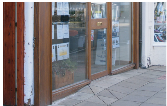
Picture 3 POOR : Stall riser
