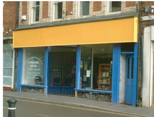
Picture 15 POOR : Oversized boxed out fascia board with no cornice or architrave or capitals to enclose it or support it. It dominates the shop front to an oppressive degree
