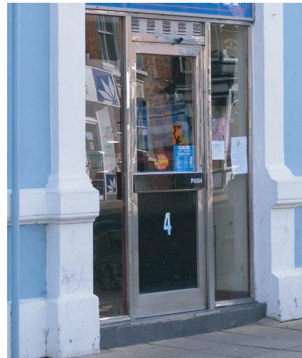
Picture 17 POOR : Door
