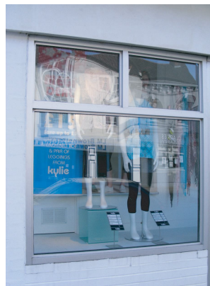
Picture 11 POOR : Mullions
