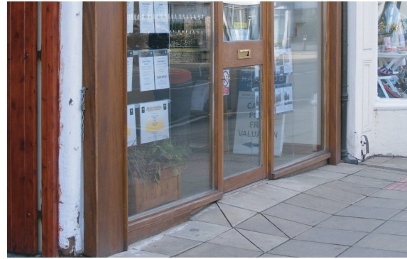
Picture 3 POOR : Stall riser
