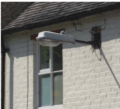
9a. Wall mounted street lighting
