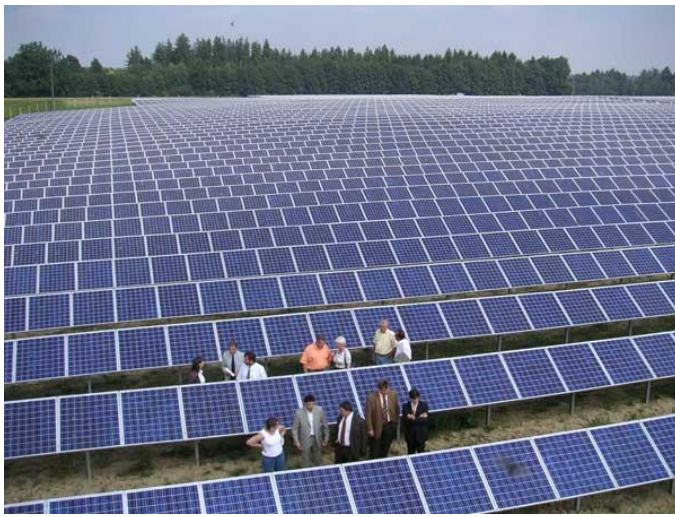
Figure 1 – UK Solar Farm
