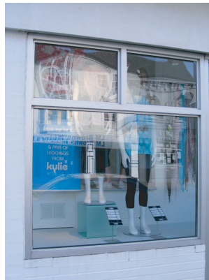
Picture 11 POOR : Mullions
