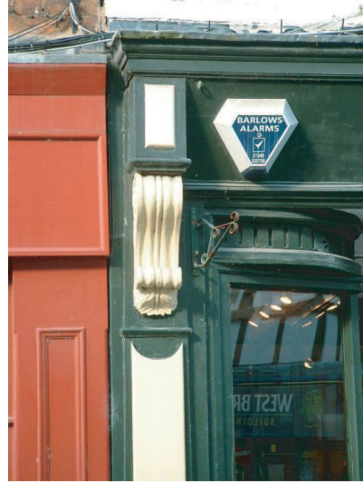
Picture 8 Good : Raised panels on the columns and bracketed capital above contrasting paint finish picks out the architectural detail
