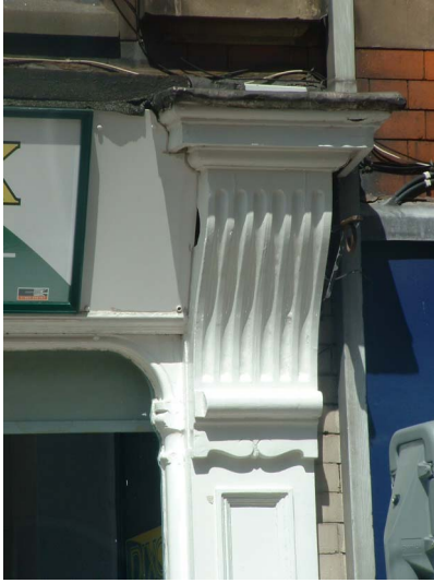
Picture 7 GOOD : Fluted capitals with a cornice at the top to give protection above a recessed moulded column
