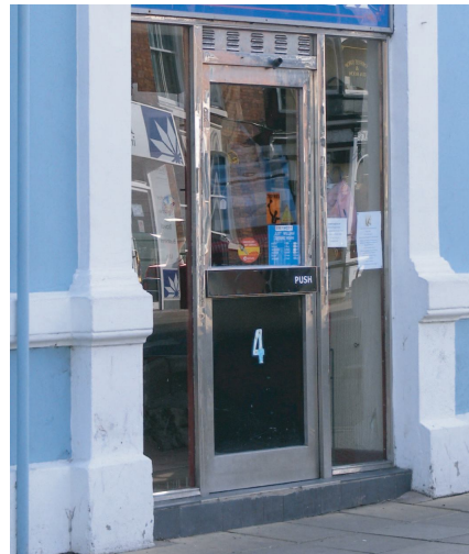
Picture 17 POOR : Door
