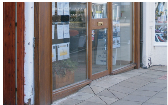
Picture 3 POOR : Stall riser
