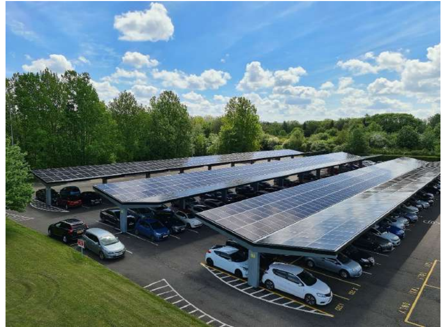
Figure 12: Solar PV Carport at Ricoh, Priorslee.jpg
